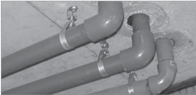
Typical Pipe Hangers
